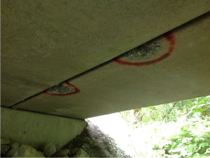
previously noted spalling concrete - has not expanded
